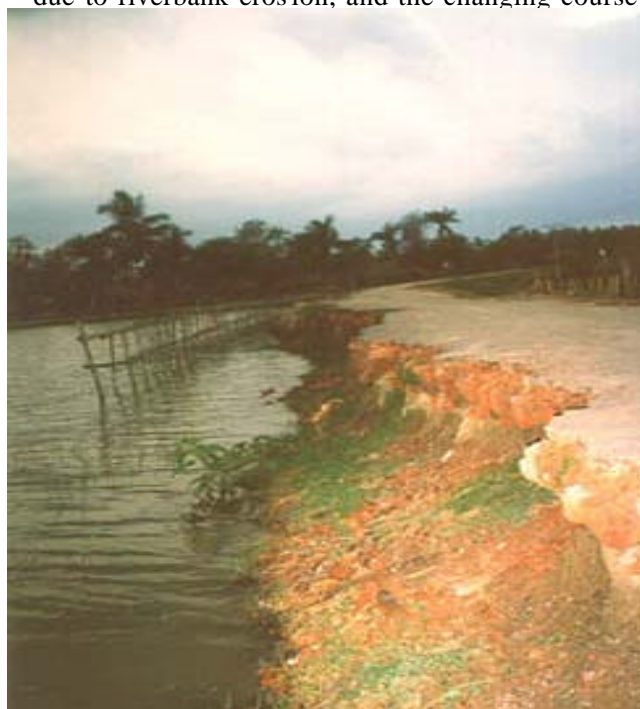
River bank erosion
